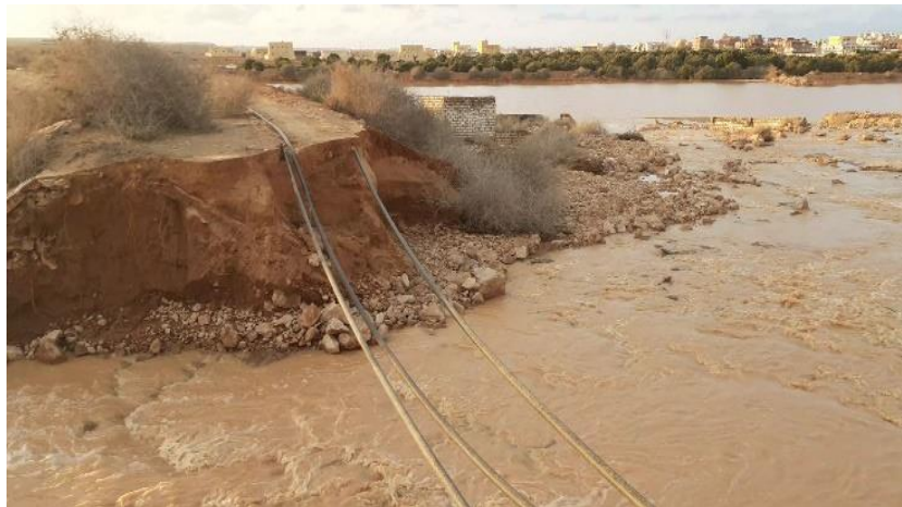
Figure 11. Collapse in the earth fill barrier
